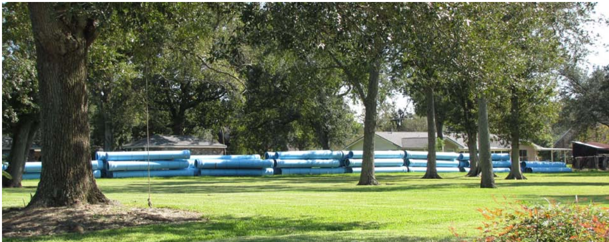
PHOTO: PVC Pipe lined up behind homes to be used to re-route the wastewater lines.
