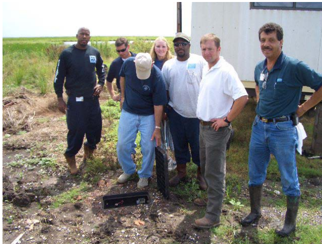
Final Inspection of the water line. Byron Williams, Jr. Plaquemines Parish Director of Public Services, Bart Peak of Wallace Drennan Inc., Robert Nockton and Paul Adams of Linfield, Hunter & Junius, Inc., Troy Phillips & Gerald Encalade of Severn-Trent, and Mary Ann Webster with Plaquemines Parish Land Department
